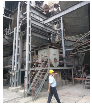
Visit to Torrent Power House at Ahmadabad for Fan Consultancy projects
